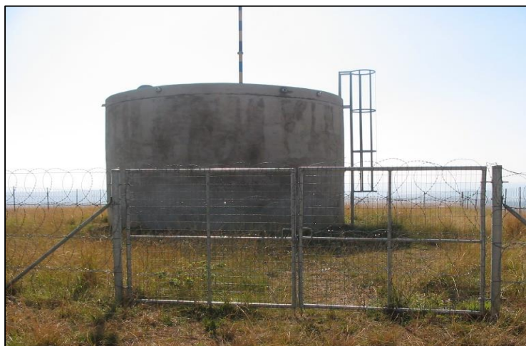
Figure 4-4: A Smaller Reinforced Concrete Reservoir
